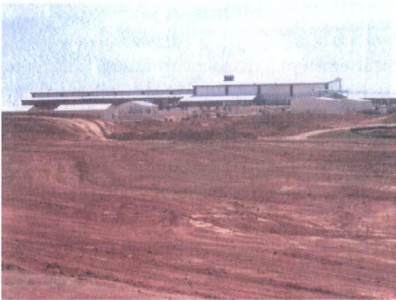
Extensive grading in progress in preparation for development of 6 large new Base facilities. Stormwater drainage patterns were the governing factor in determining new facility locations.
